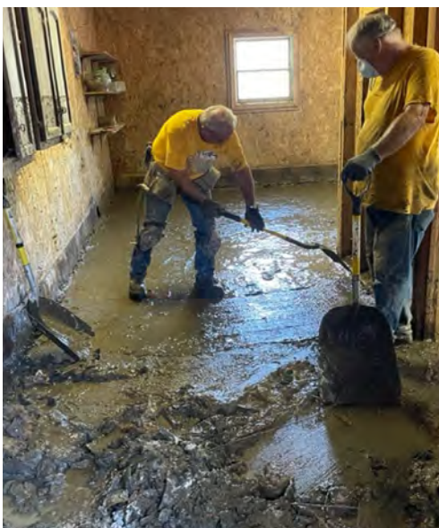
Ohio DR Teams shovel 3-5 inches of mud and remove everything from inside a flooded home in Kentucky.
